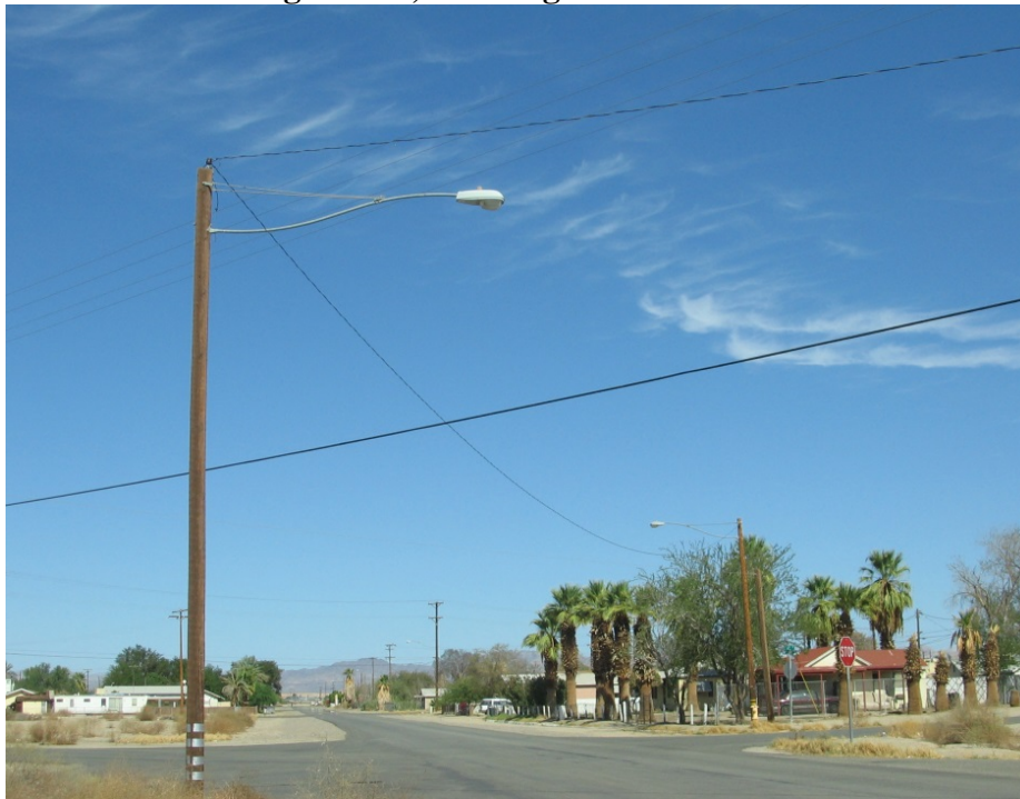
Existing streetlight located along Main Street
